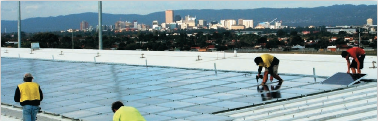
Solar panels on T1 rooftop
