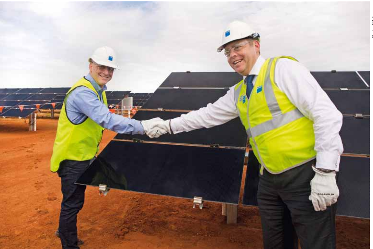
AGL CEO Andy Vessey with New South Wales government minister Anthony Roberts at the installation of the final module.
